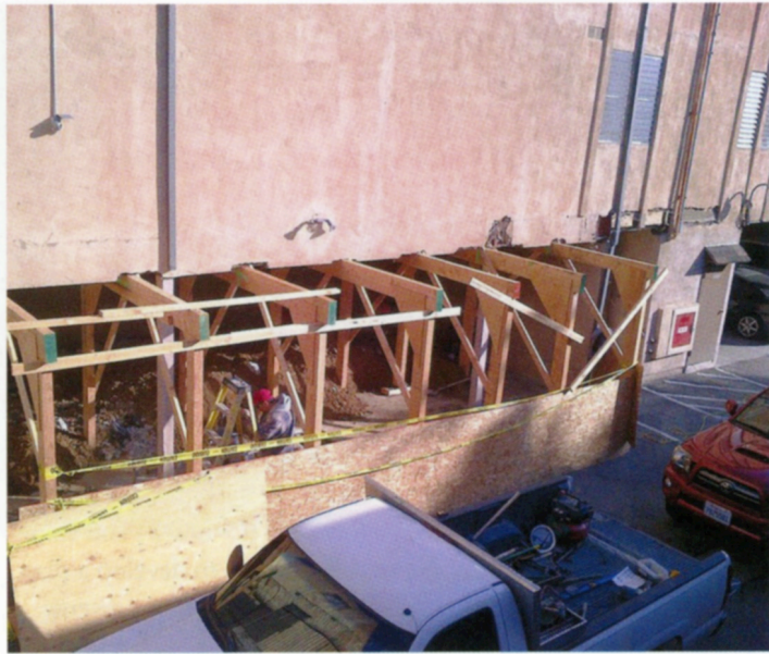
Soft-story buildings are vulnerable to earthquakes. In Los Angeles, many are being reinforced.
